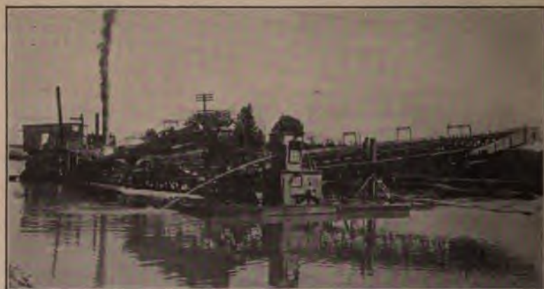
View of Elevator End of Steel Pontoon Dredge Operating on New York State Barge Canal.
